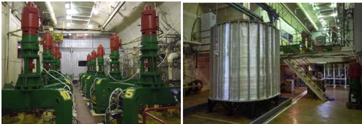
A view of the GGNT(left) and 2 zone installation BEST(right)
