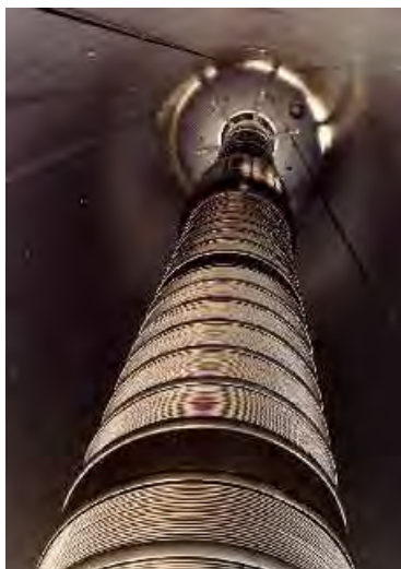
Figure 15.2: Inside the tandem
